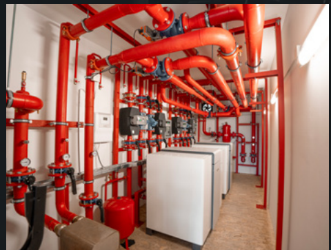
water/water heatpump center inside
